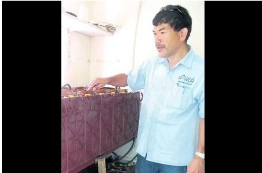
Managing Director of Alternative Power Sources, Damian Lyn looks at the battery backup system at Chong's St Mary residence. (Photos: Alesia Edwards)
